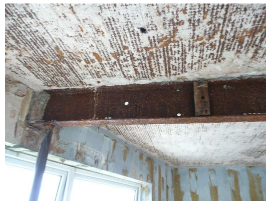
Corroded Support Beam and Slab Reinforcement
